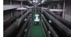
Power facility patrol
